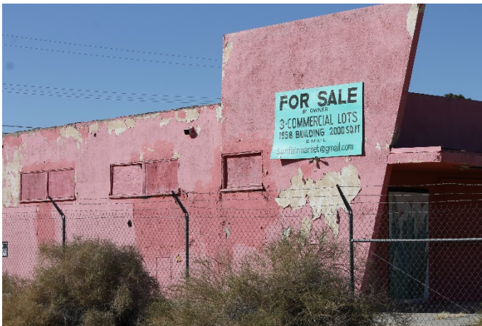
A downtown business improvement district (BID) can help to promote vacant properties and increase value in the area. Photo source: Michael Baker International
