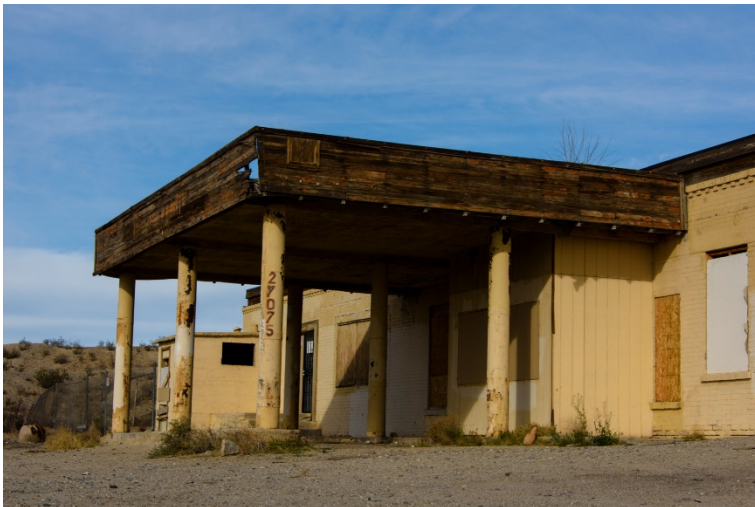
Vacant property in Helendale. Photo source: Michael Baker International
