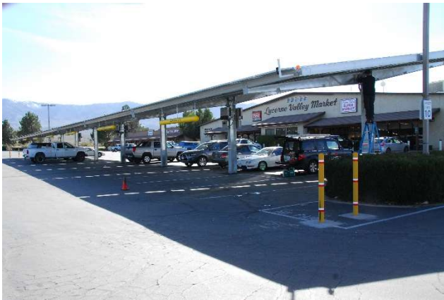
Solar Panel/shaded parking that is installed in front of the Lucerne Valley Market. Photo source: Cal Poly Pomona
