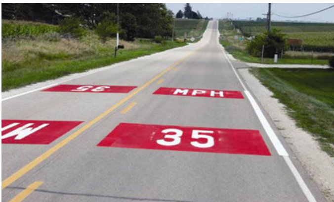
Experimental speed markings with red background have been shown as effective in reducing vehicle speeds. Photo source: Federal Highway Administration (FHWA) Research and Technology
